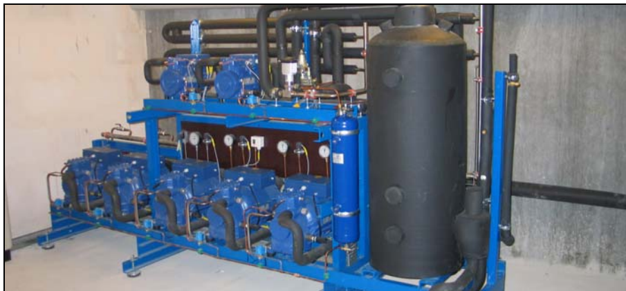
A picture from the installation
